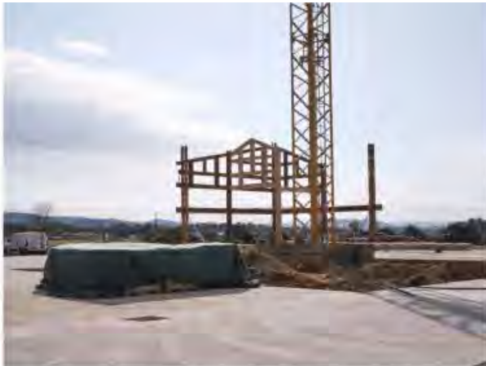
At his home in Portugal, Ai is building a replica of his Shanghai studio (torn down by the Chinese authorities in 2011), working with local construction workers and using traditional Chinese techniques (Image credit: Jermaine Francis)
